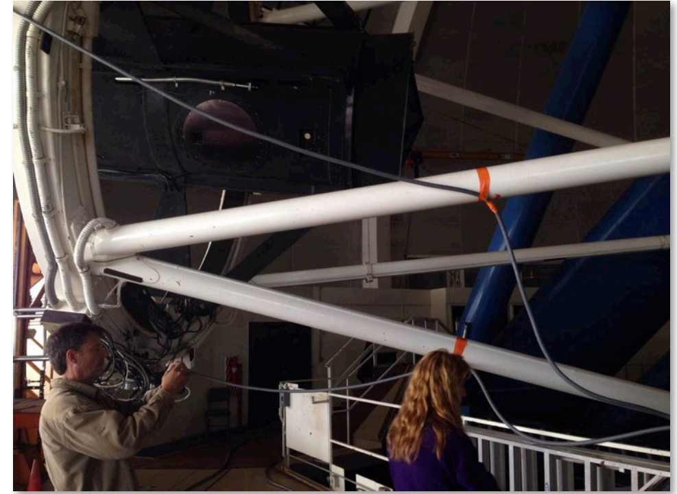
KPNO engineer Derek Guenther (left) and safety officer Tammie Lavoie(right) studying process for stringing fiber optic cables from prime focus down the telescope truss.
