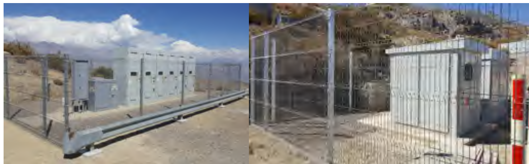
Pachón sub-station safety fences
