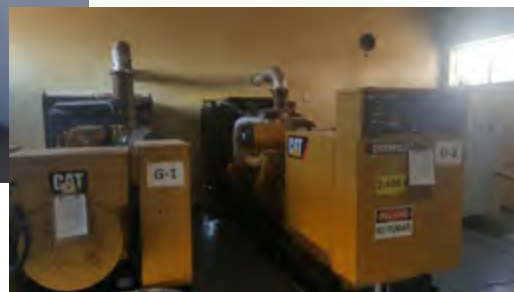
Dual redundant generators
