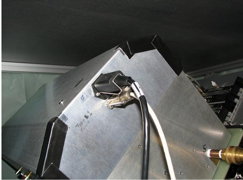
Fig. 7. Back of the monsoon crate showing C1 AC connections (black cable) and the C2 ICS control connection (white cable).
